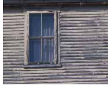
↑ Large pane window requiring maintenance or repair. East Angus.
